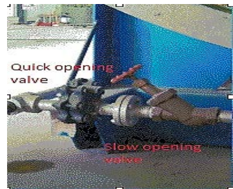
Figure 46 Boiler Blowdown valves (Courtesy of Eneritech-Philippines)
