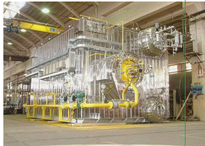
Figure 20 - Installed watertube boiler (LBL Italy) (185)
